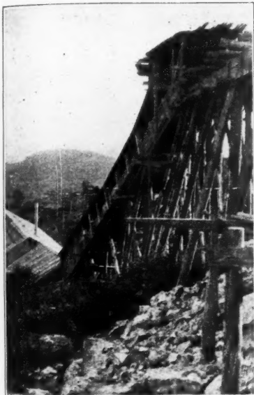
Point Where Rock Is Dumped to Crusher
